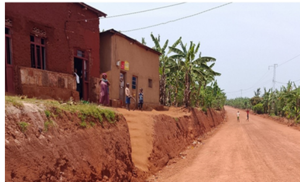
Houses are very closer to the vertical cliff caused by road construction cuts (Ngoma District)
