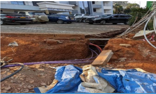
Cables near public areas without proper safety controls (Nyarugenge District)
