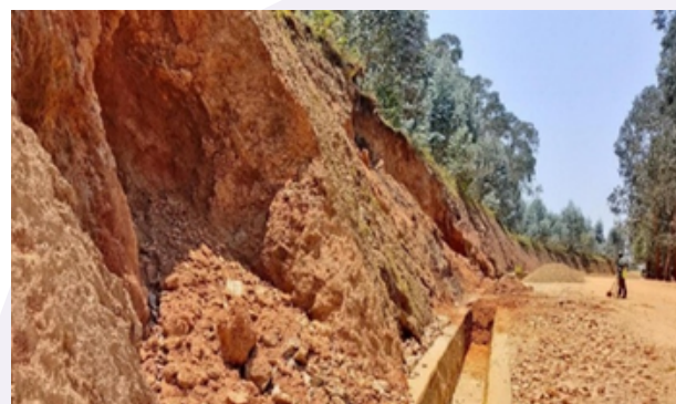
Rutsiro District: dirt slides along new roadway
